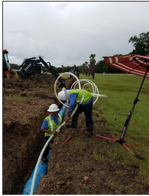
Photograph 4: 2-inch Trickle Feed Pipeline
